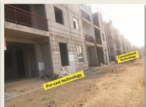
Visible difference between quality of villa constructed using pre-cast and conventional technology at GGL
