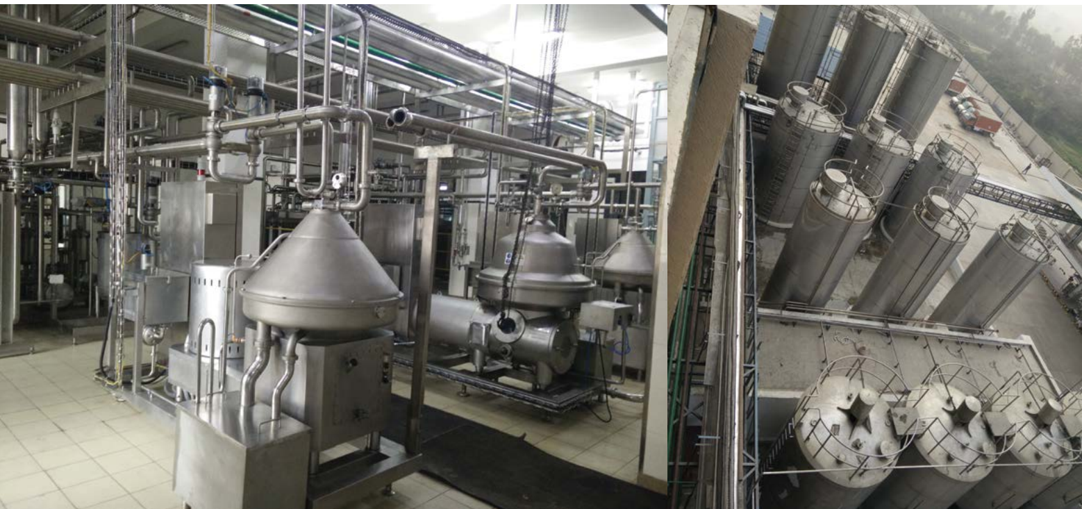
Pictures of Kwaliti Dairy's Faridabad factory; Dairy industry requires very high capex
