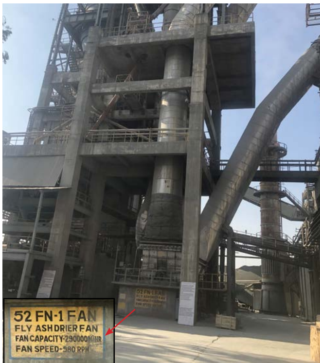
IKN Cooler and fly ash drier at a cement plant
