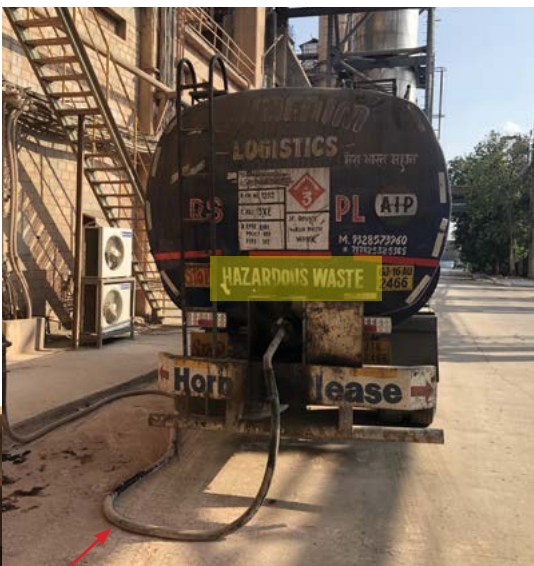
Fuel pipe connecting the tanker directly to the fuel disposal system of the plant
