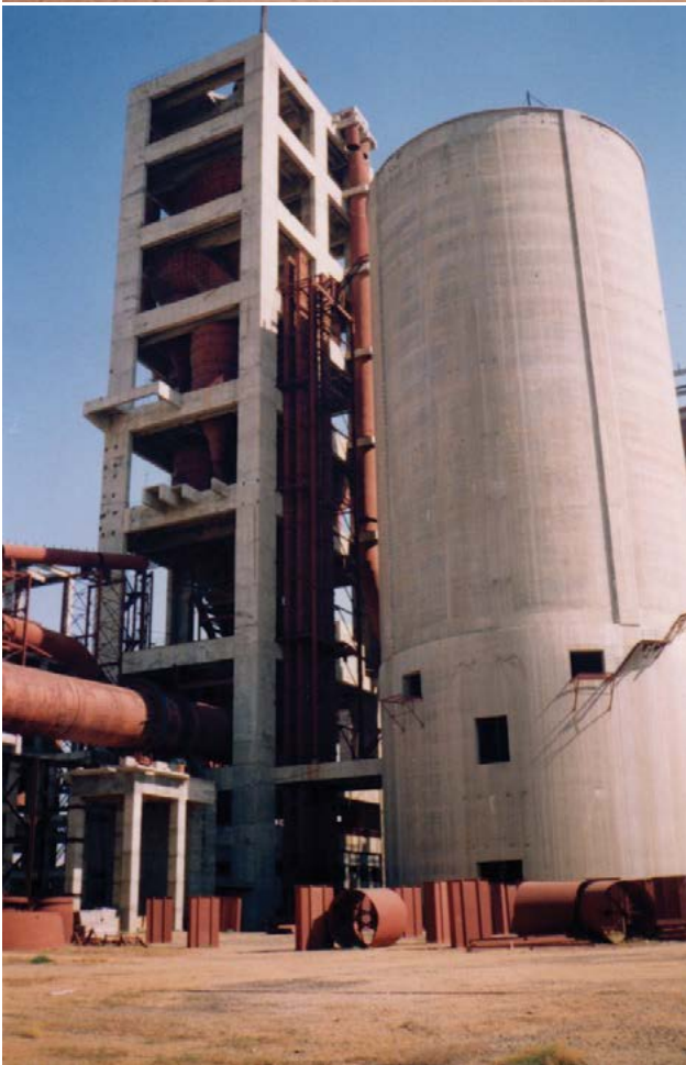
Sanghi Industries plant in 1999 when 70% construction of the plant was already complete.
