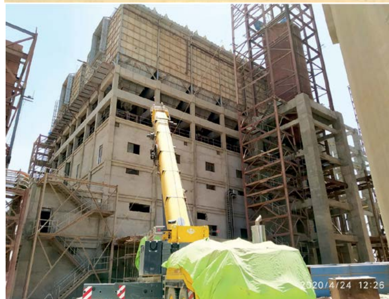
A glimpse of construction state of Sanghi Industries second unit, as on 24 th April 2020.
